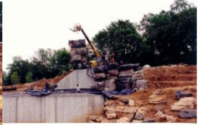
The rock sections are lifted into place, bolted together and anchored to the wall and pad.
