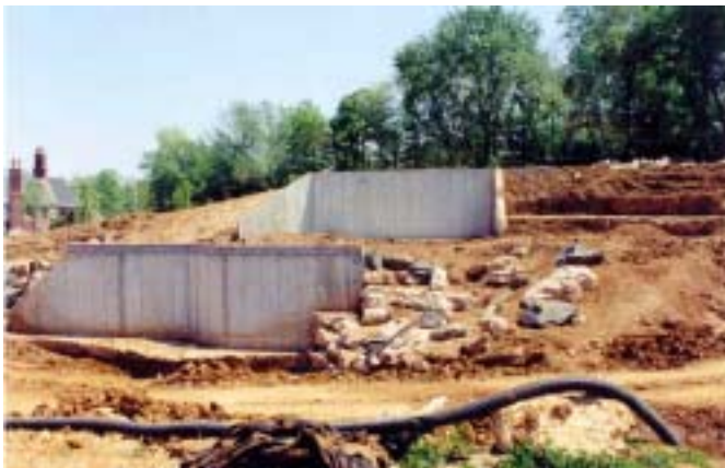
A concrete retaining wall with a 3 - 4 foot pad is poured in preparation for the artificial rockscape
